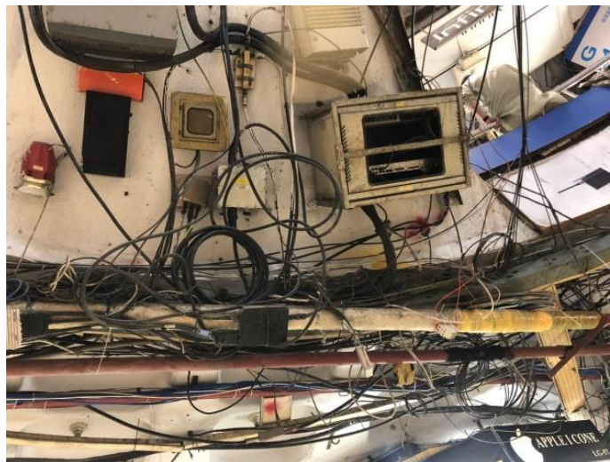
Figure 14 Infrastructure Condition of Hafeez Center
