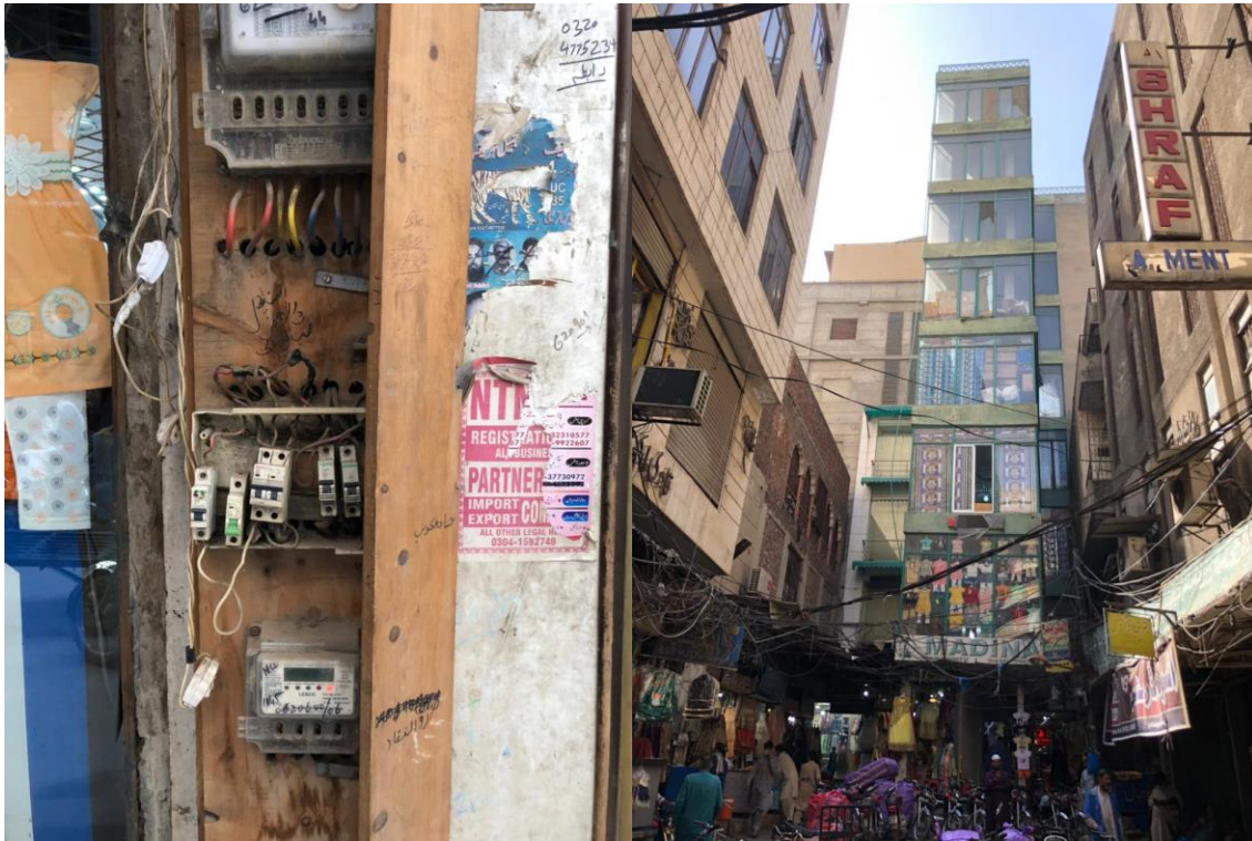
Figure 12 Infrastructure Condition of Shah Alam Market
