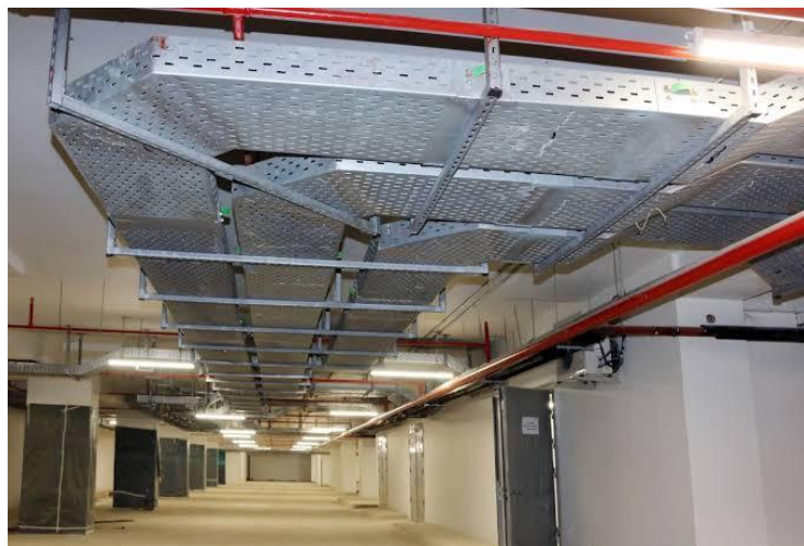
Figure 13 Infrastructure Condition of Emporium Mall
