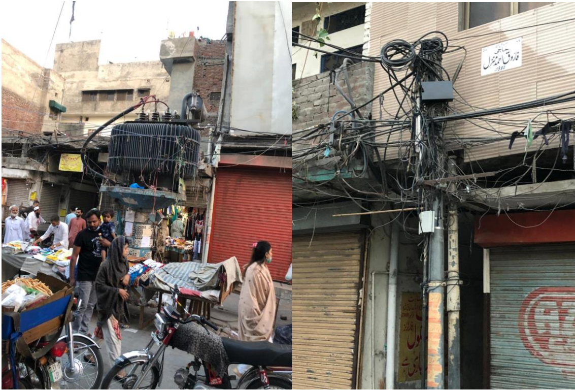
Figure 11 Infrastructure Condition of Baghbanpura Bazar
