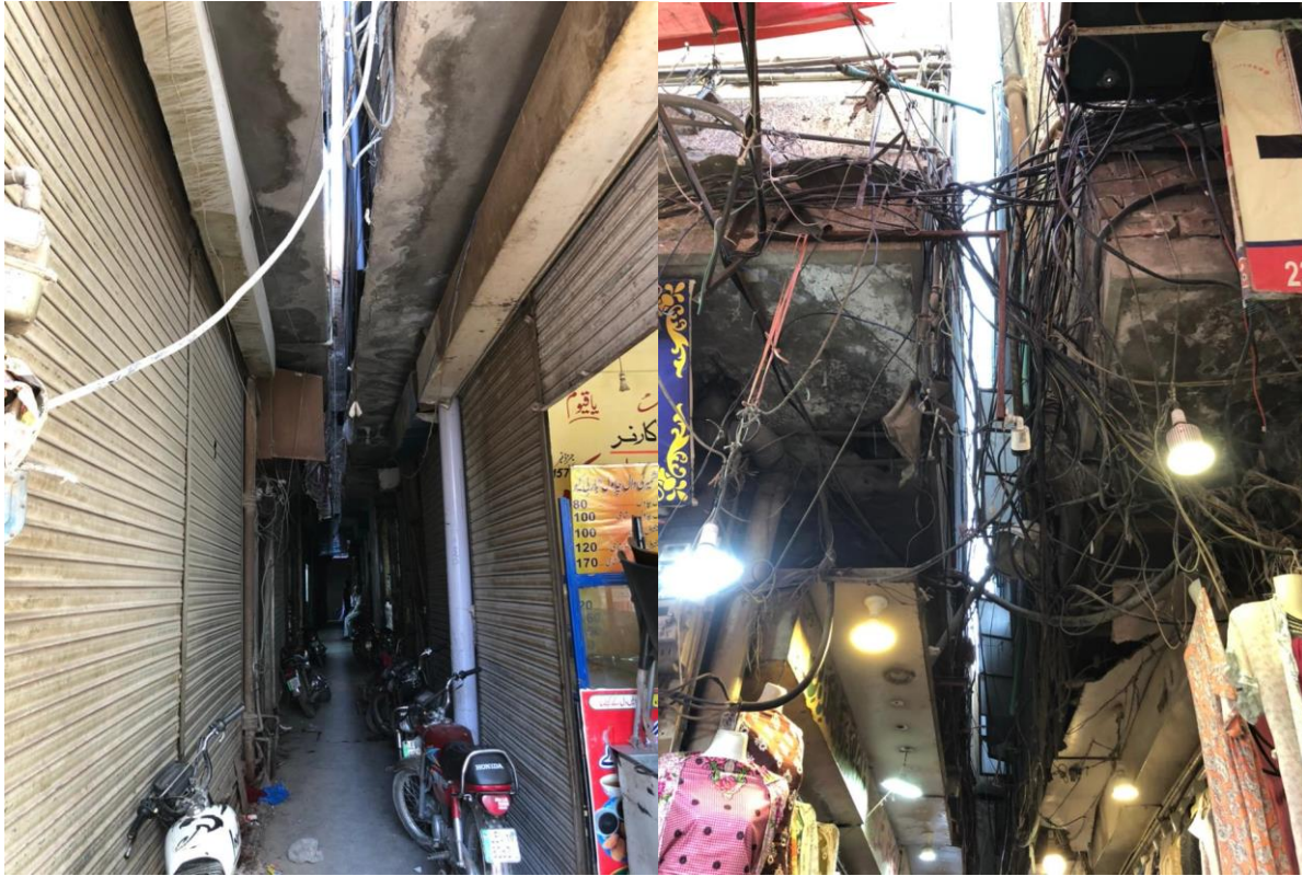
Figure 10 Infrastructure Condition in Icchara Bazar
