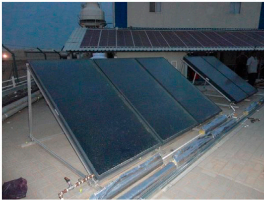
Fig. 8. Flat plate collector array aperture area 11.85 m 2 .
