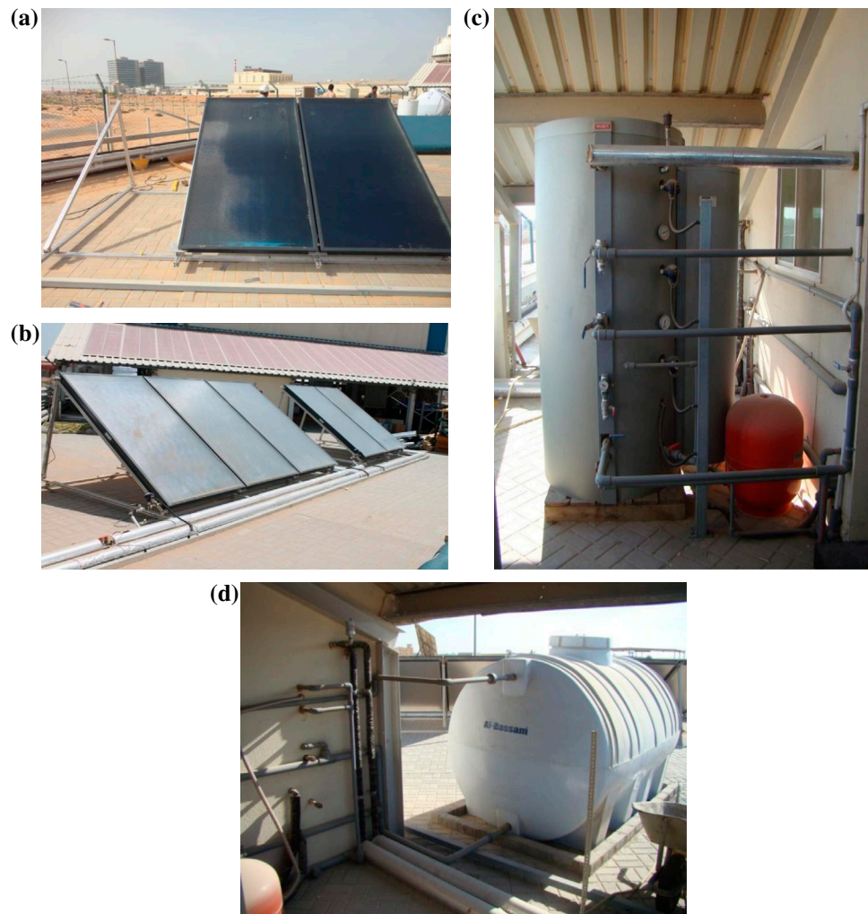
Fig. 5. (a) Installation of flat plate collector plates, (b) orientation, placement and angle orientation of collectors, (c) stratified thermal storage tank with piping circuits, and (d) cold water storage tank (municipal water supply).
