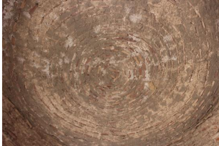
Figure 50: Arcuated System of Brick Masonry for Domical Construction followed in Shalimar Gardens
