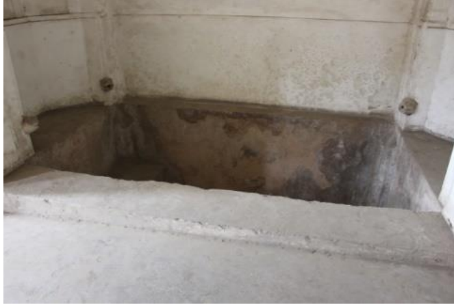
Figure 39: Reservoir for Water of Desirable Temperature
