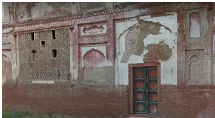
Figure 55: Perforated Terracotta Lattice Work on Exterior Wall of Shahi Hammam with Pacca Kali Plaster
