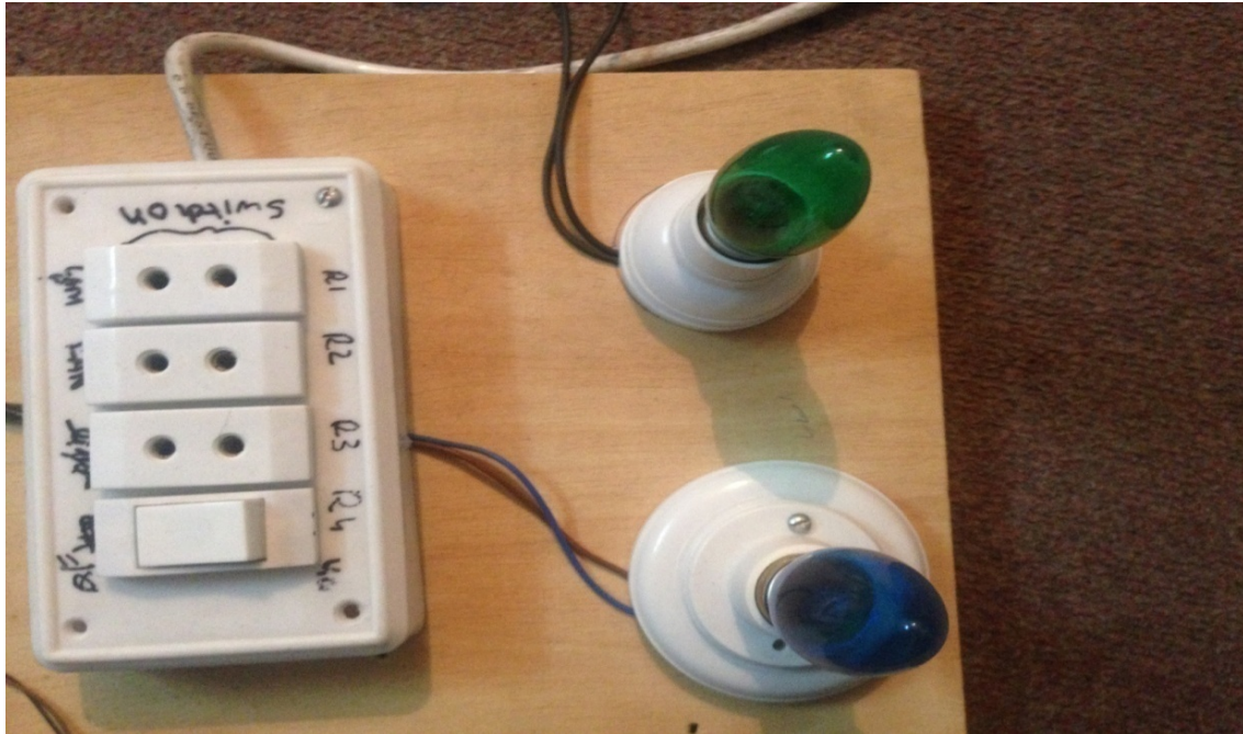
Figure 21: Switch Board and Load Connection
