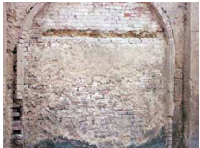
Figure-7: Poor conservation of Shish Mahal
