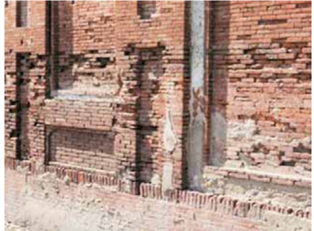
Figure-1: Deteriorated bricks.
