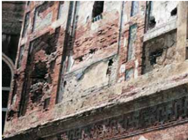
Figure-2: Deteriorated patches of bricks.
