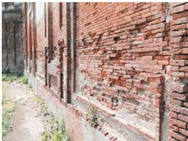
Figure-4: Erosion of mortar from brick wall.
