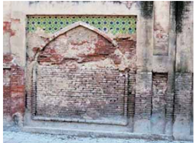
Figure-6: Defective plaster rendering of Shish Mahal
